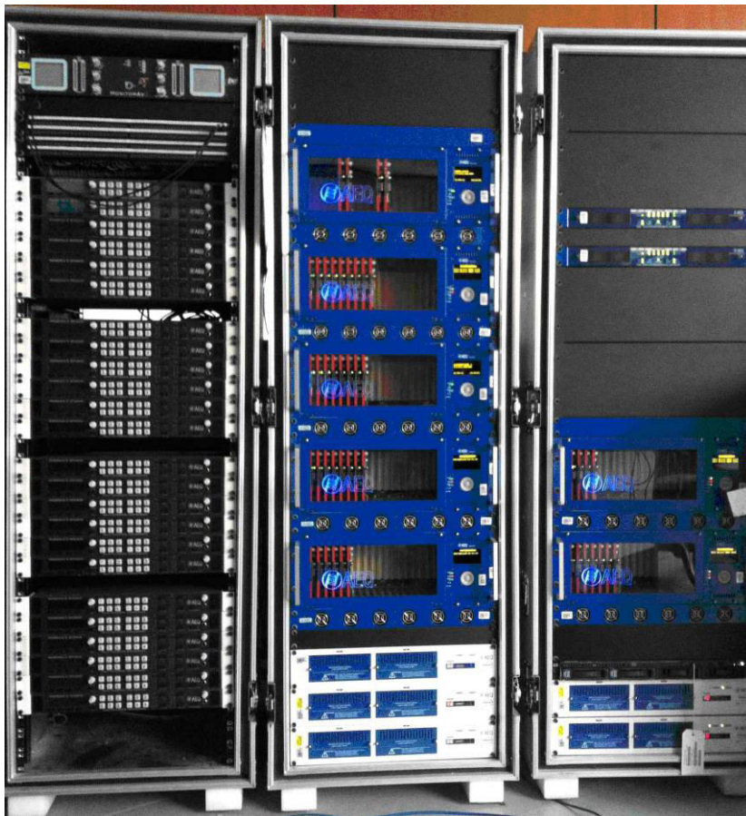
Figure 2: EBU switching centre, showing the AEQ TITAN frames (right), Interface Frames (center) and 24 Phoenix Studio for international circuits distribution, ready to be installed in London.
